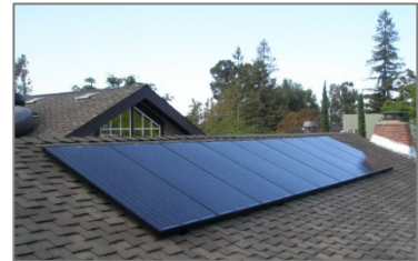
Figure 3.2 Building-mounted solar energy system
