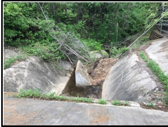
Figure 2 Channel Wall Failure and Debris Blockage
