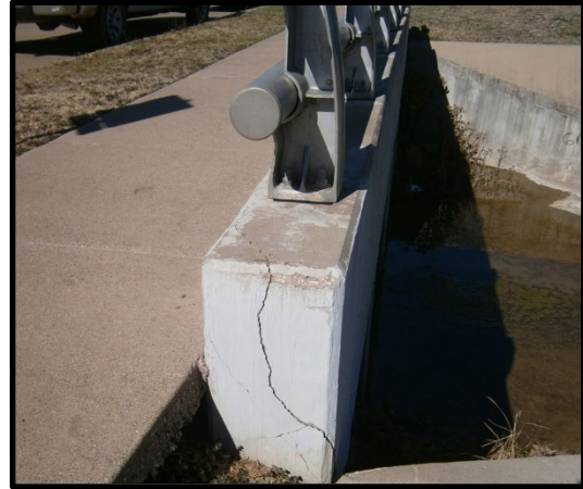
Figure 5 - Headwall Cracks Identified During Channel Inspection
