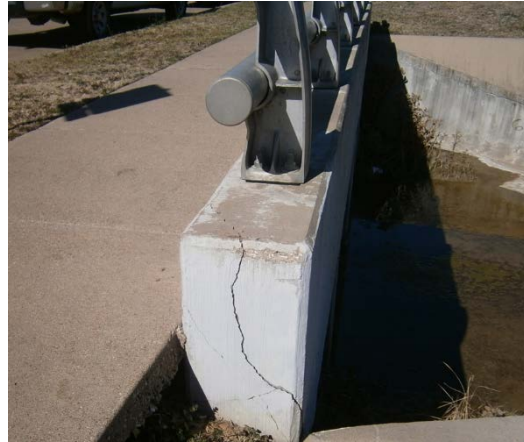
Figure 2.2.4 Headwall Cracks Identified During Channel Inspection
