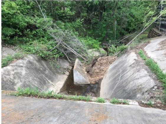
Figure 2.2 Channel Wall Failure and Debris Blockage
