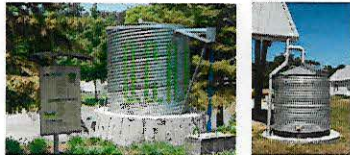
Shade Structure with Rainwater Harvesting Cistern
